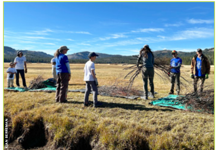
Lower Lacey Meadow: It takes all of us to get the work done! Volunteers come together to collect willow cuttings and make debris jams and willow wattles.
