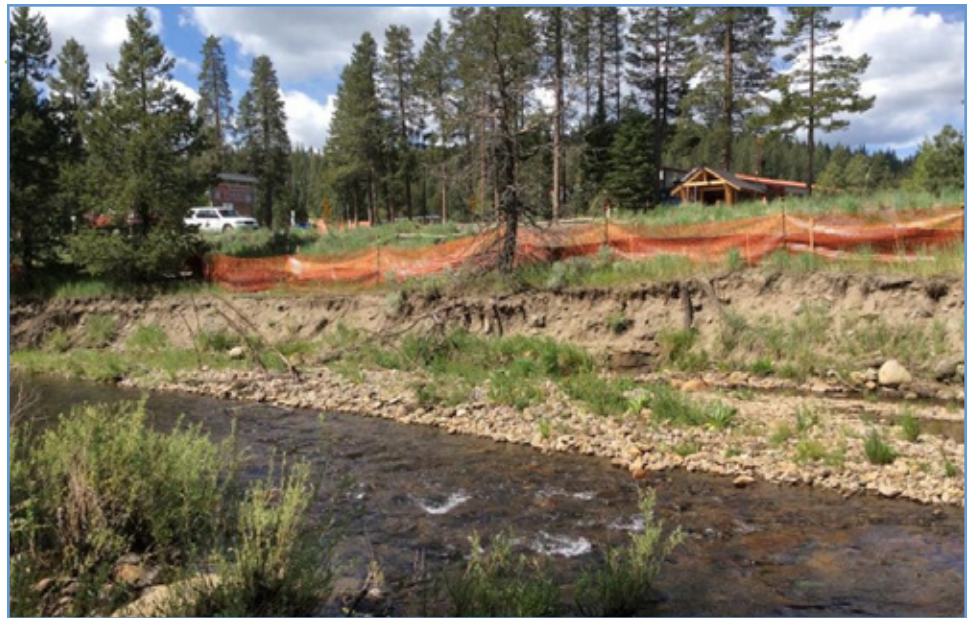
Severe erosion on the right bank, fine sediment loading, and poor habitat quality are present at a site along Donner Creek.
