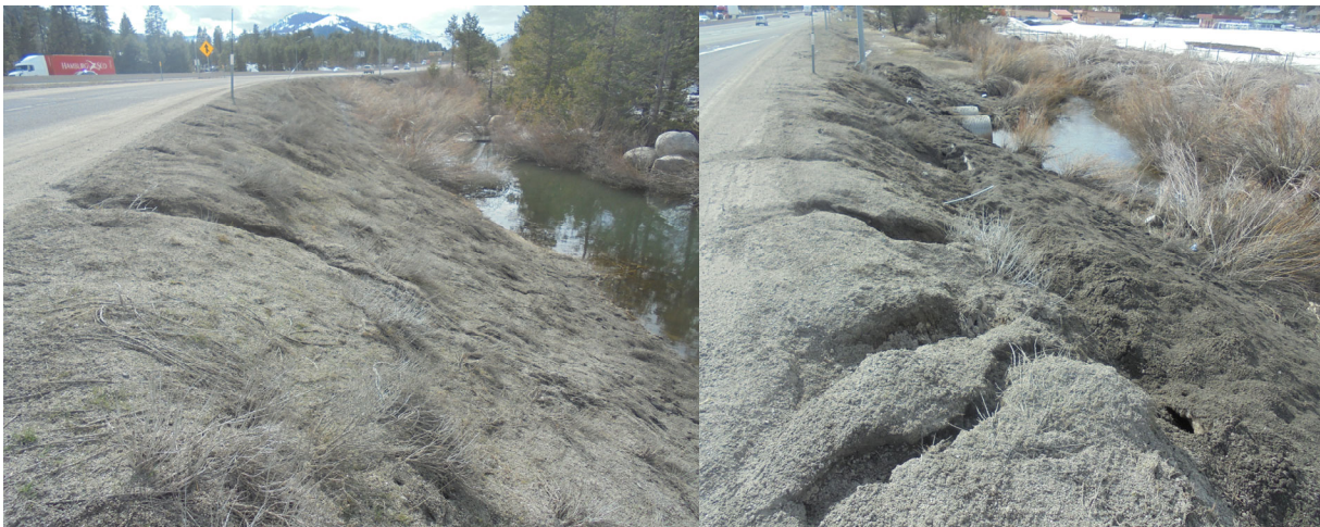
Figures 5 and 6. Site 3 drainage looking westward. Gullies forming along shoulder drainage.
