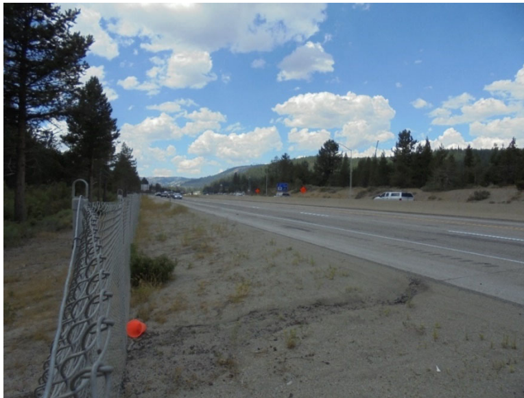
Figure 2. Site 4 rilling from freeway runoff, looking west; grass-lined swale with check dams proposed along south side (left) of fence.
