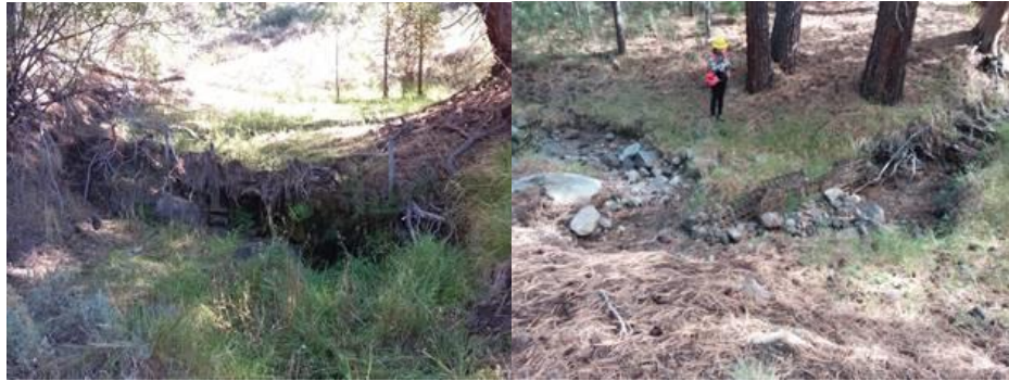
Figure 10. Erosion of grade control structures.
