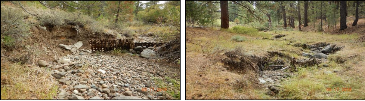
Figure 6. Failing Marston Mat grade control structures in Canyon 4.
