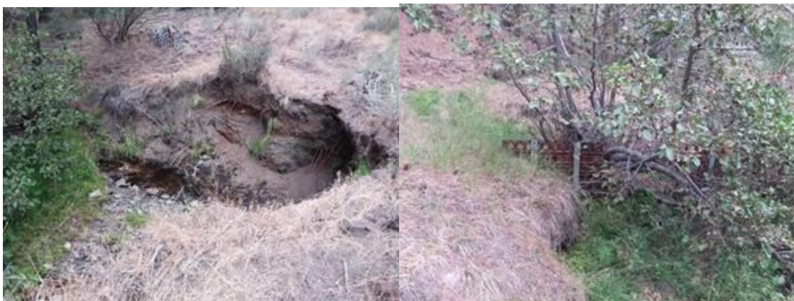
Figure 9. Erosion from the stream cutting around the grade control structures shown above.
