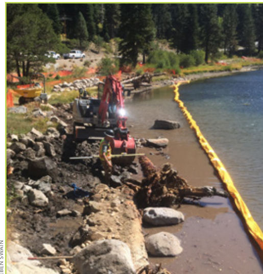
Left: The First 4 Miles Restoration Project between Tahoe City and River Ranch during construction.
