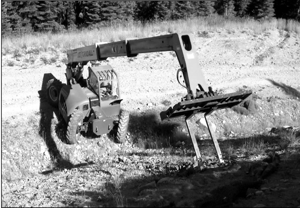
Figure 4: Infiltration tine-type of treatment in hard to reach areas using a reach forklift.
