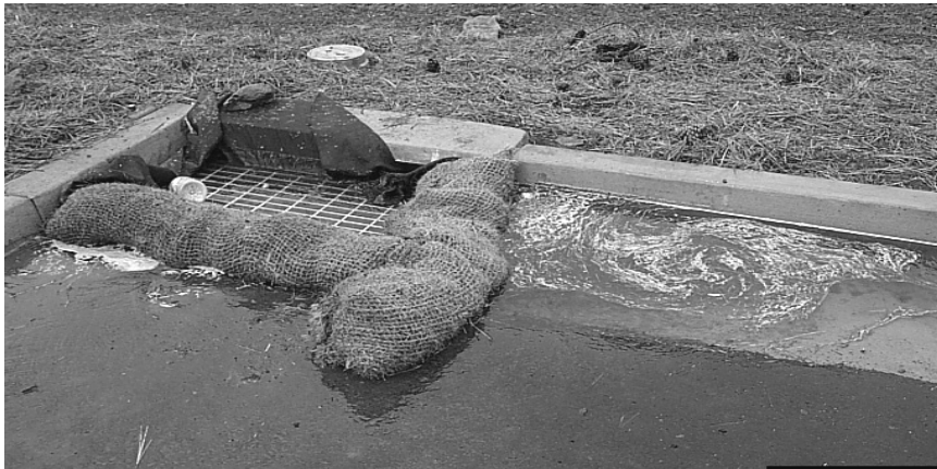
Figure 1b: Drain Inlet with Pine Needle Wattles and Filter Fabric Installed around Drain Inlet
