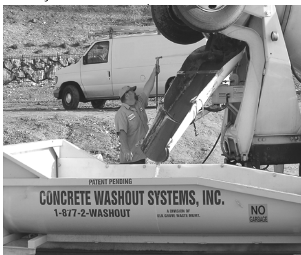
Figure 1: Examples of a Concrete Washout systems used on Northstar construction
