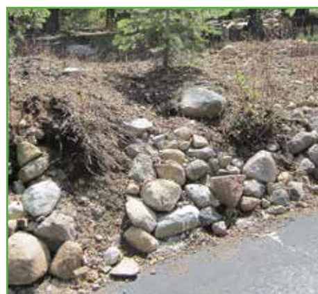
Sediment from an eroding bank at a Donner Lake property will eventually run into the lake, having a significant impact on water quality.
